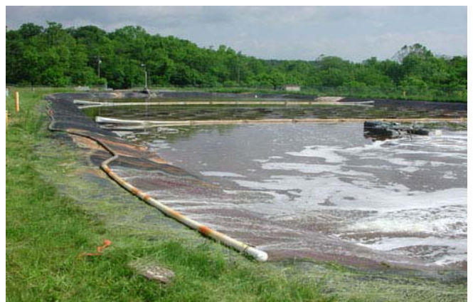
Secondary Cell (Before), Surface Aerators, Plant-Based Filtration Only
